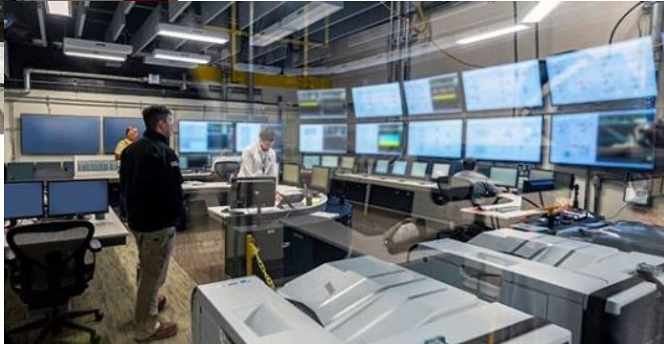
Vogtle Unit 3 Control Room
