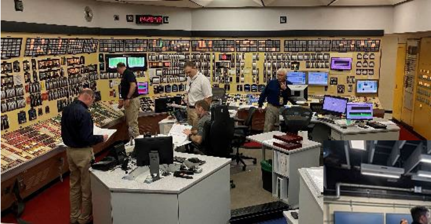
Vogtle Unit 1 Control Room
