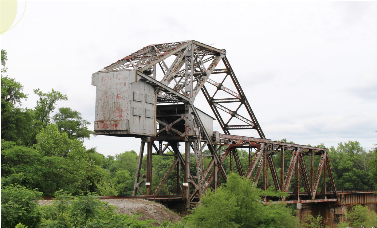
The Doctortown Trestle is the only still-active railroad bridge that spans the Altamaha River.
